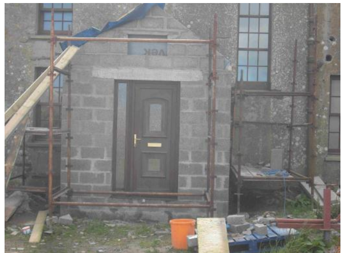
New porch with temporary door. The hole left above the door is for a piece of sandstone to be inserted after it has been carved.
