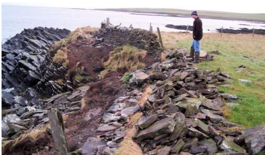
The dejected owner surveying the damage where part of the dyke below Hescombe was washed into the field by heavy seas during a south-easterly gale.
