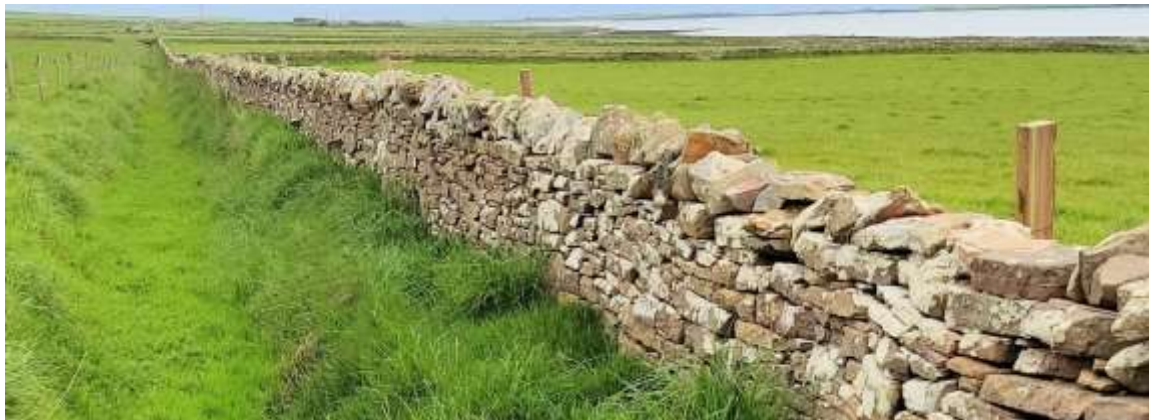
This ditch was dug and then the dyke erected on top of the excavated spoil.
