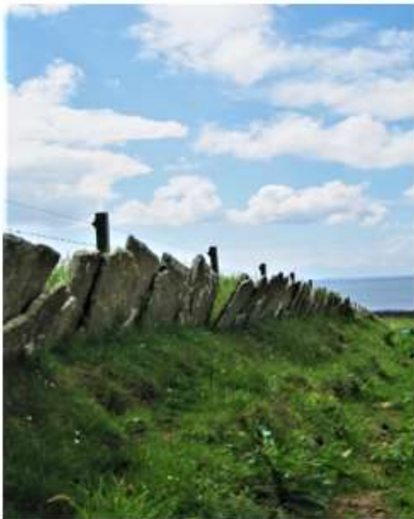
A flag fence, still in remarkably good condition after more than 150 years.
